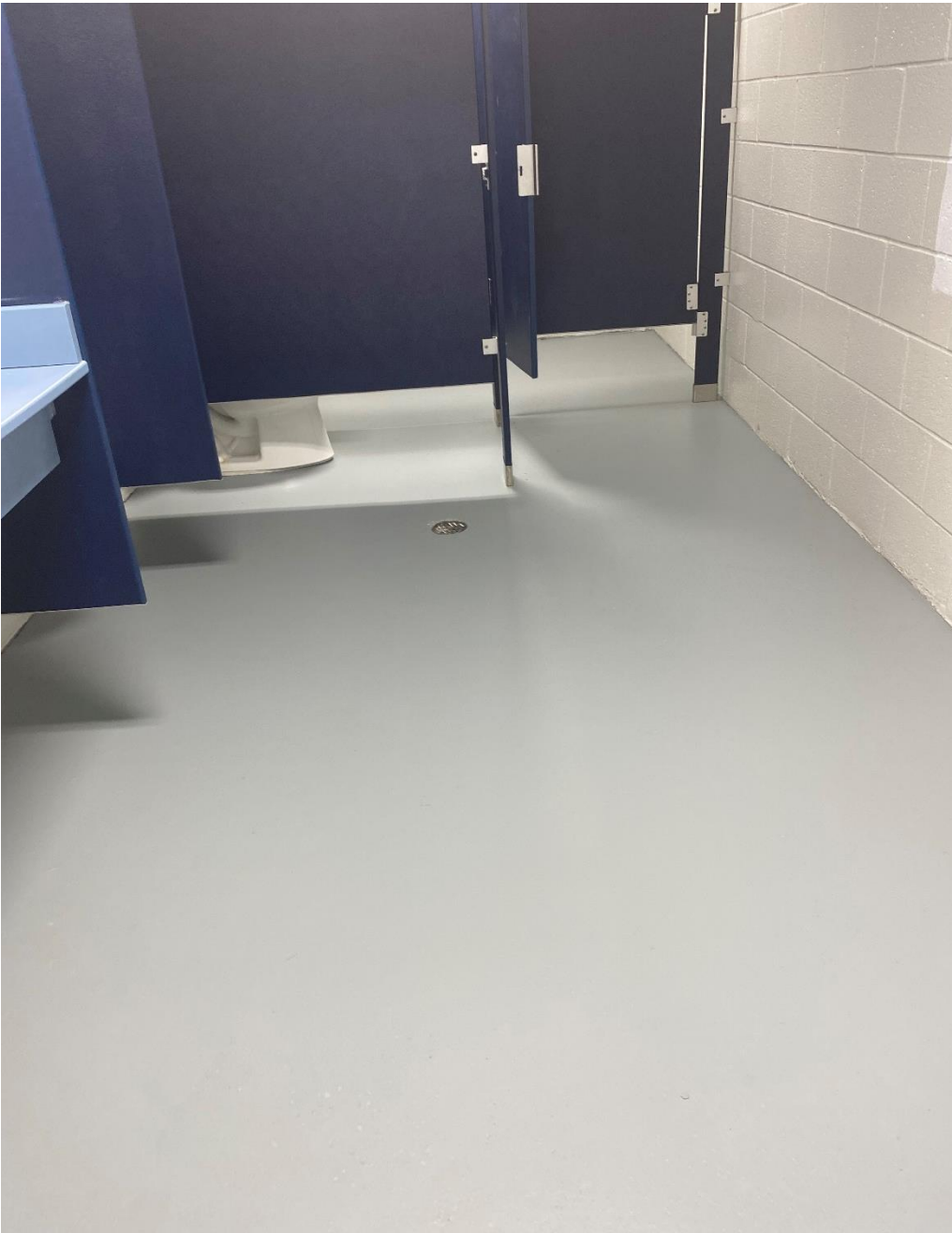
Concrete floors were painted in both men's and women's bathrooms at Brianna's Park and Memorial Park.
