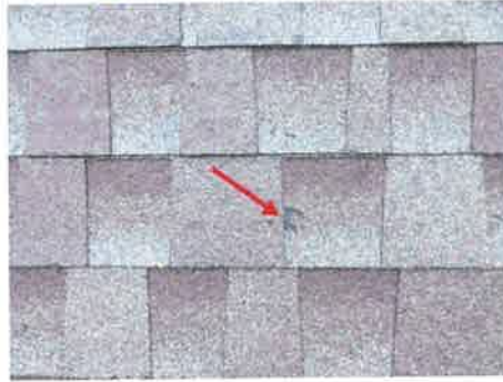
Potential Hail Damage
