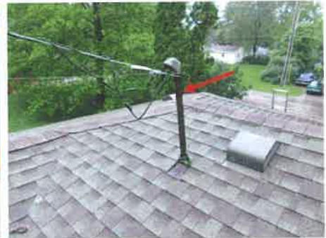
Movement at service mast
