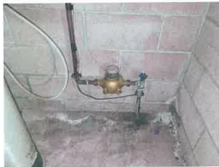
Main Water Shutoff
