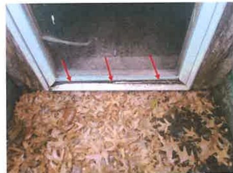
Rotting at egress window
