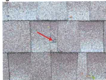
Potential Hail Damage
