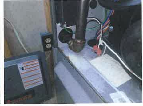
Dry Staining in Furnace
