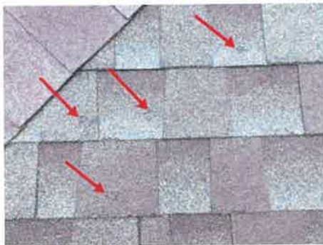
Potential Hail Damage
