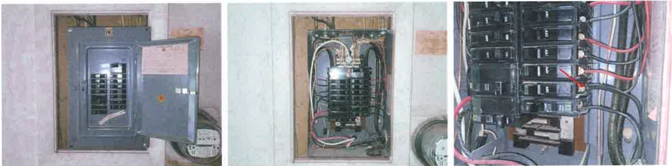
Multiple Wires at Breaker
