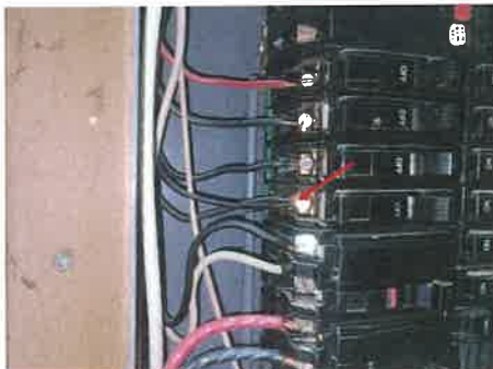
Multiple Wires at Breaker
