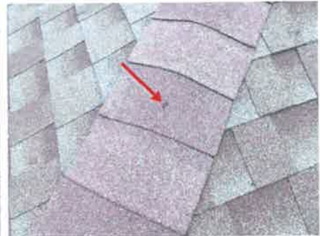
Potential Hail Damage
