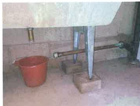
Disconnected drain line
