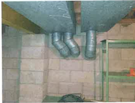
Ductwork under garage floor??
