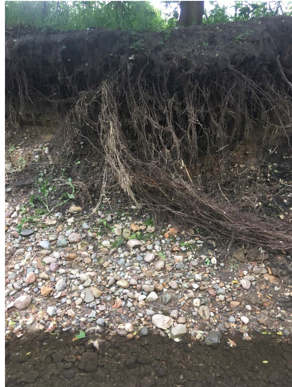
Figure 9. Exposed tree roots from incision and undercutting.
