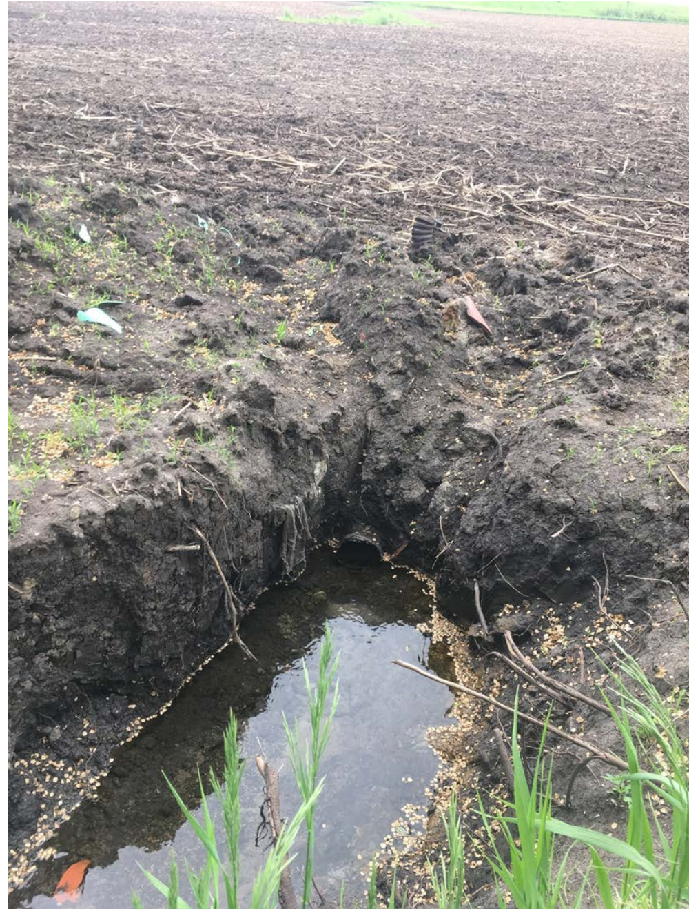
Figure 13. Tile drain outfall (center picture at water line) and associate gully erosion.
