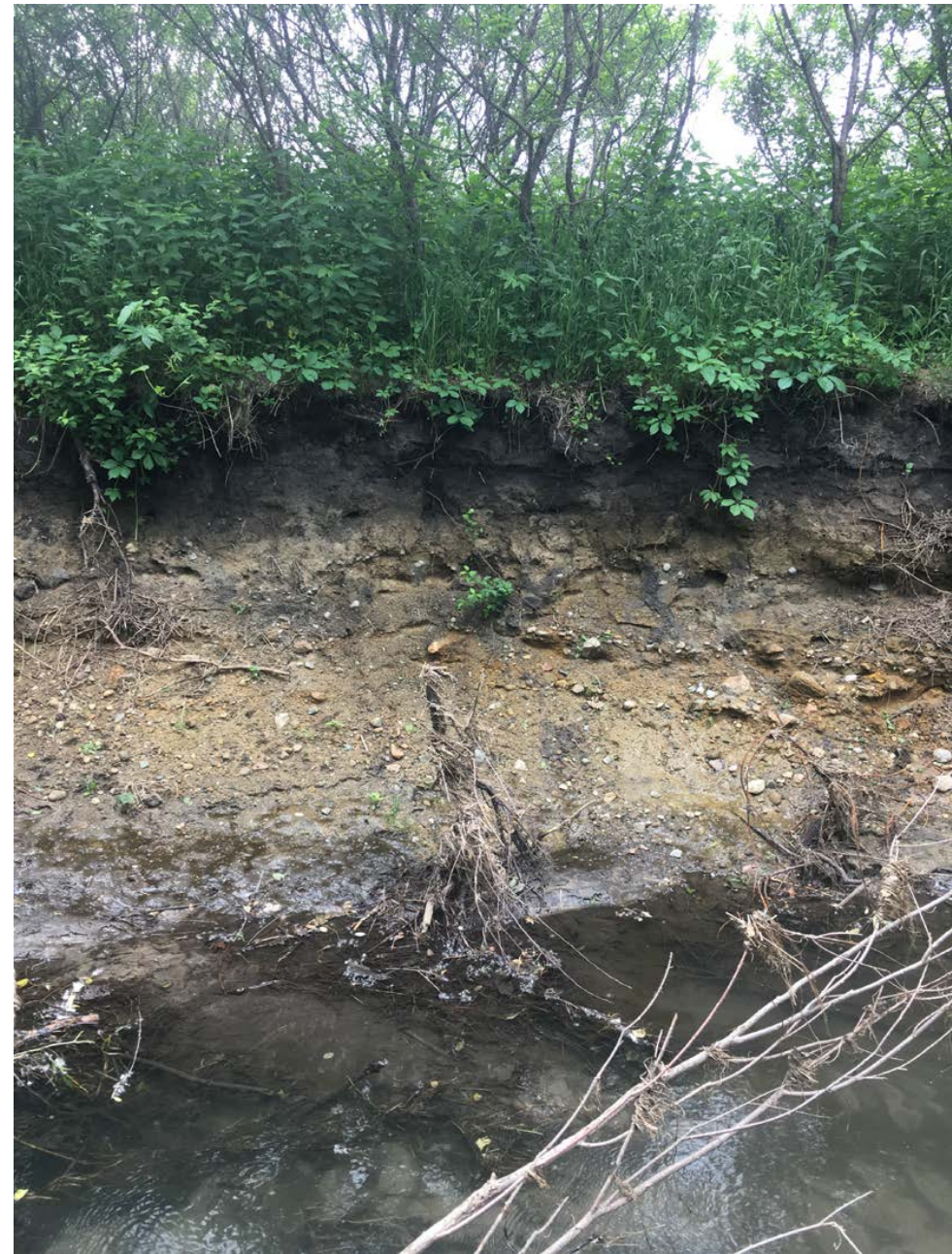
Figure 5. Typical bank soil profile showing top soil, sandy soil, and clay with gravel at the toe in this case.
