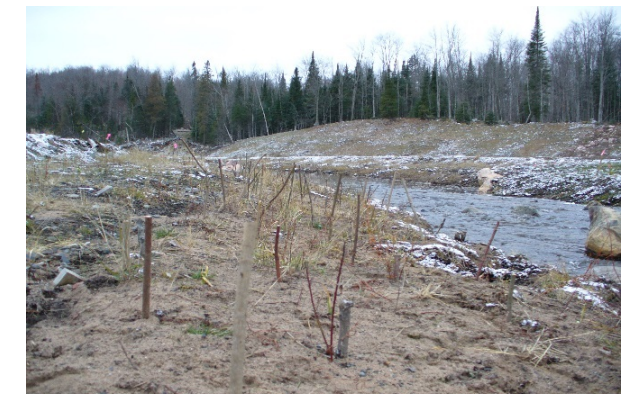
Photo 12. Live stakes installed in late autumn on Dead River, MI. Source: Collins & Baker Engineering
