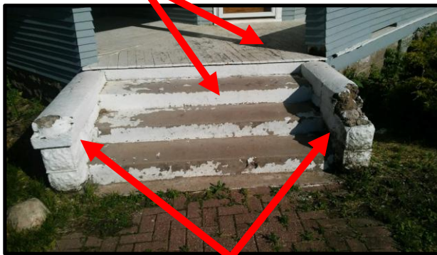
Crumbling Front Steps
