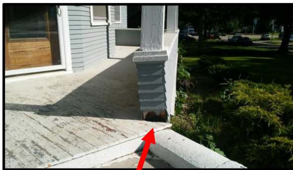
Sagging Porch Post / Wood Rot
