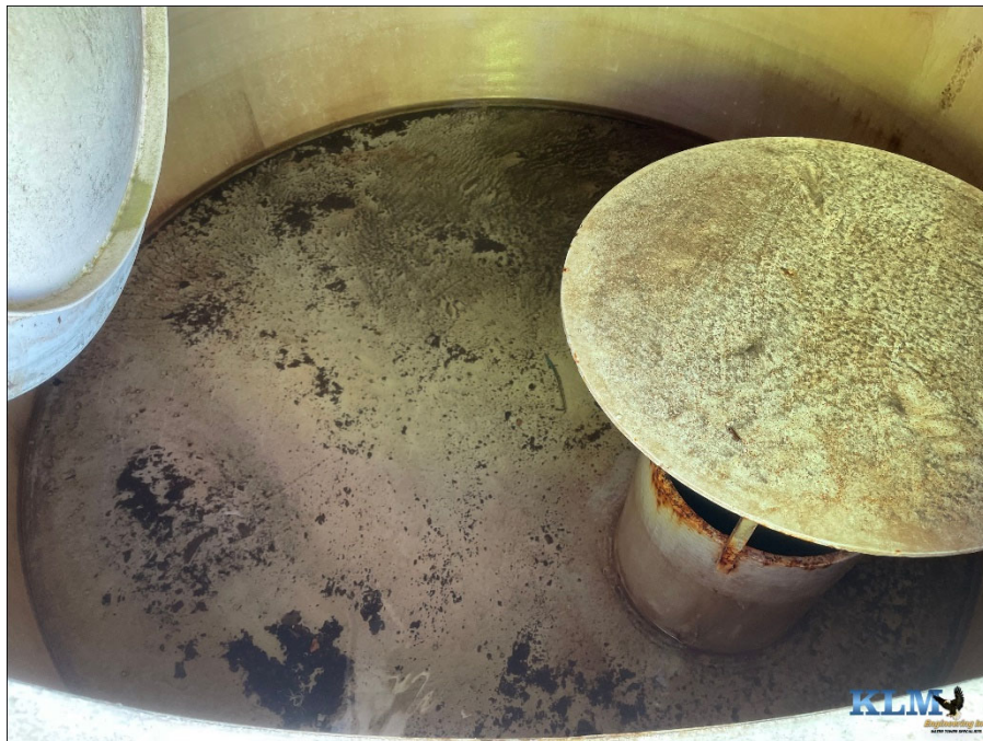
Photo No. 14 Bottom of wet riser
