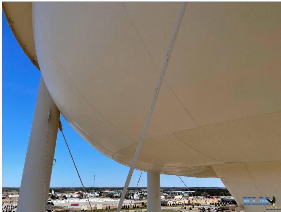
Photo No. 30 Bowl coating conditions
