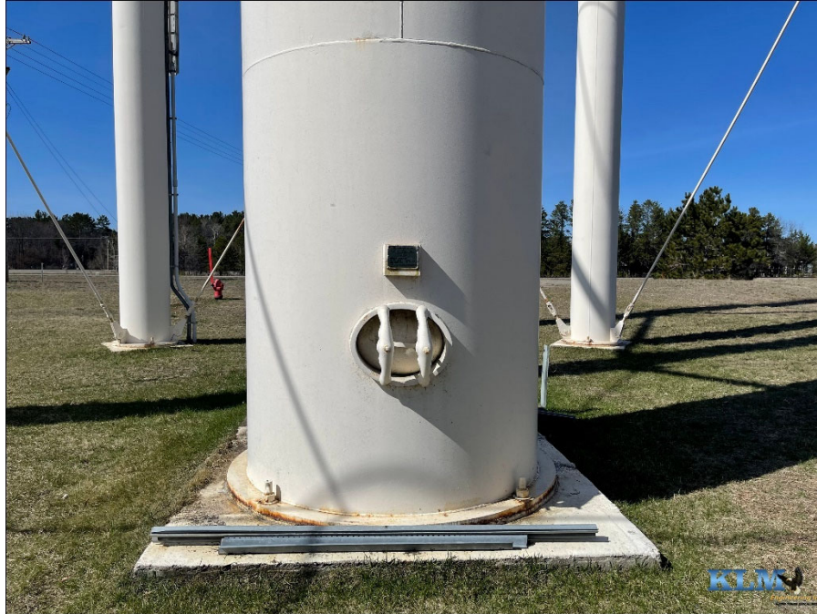
Photo No. 35 Base of wet riser
