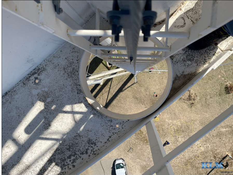
Photo No. 29 Column ladder
