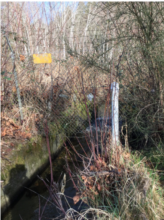
Graphic 3. Fishway Downstream of Outfall
