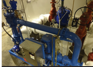
Piping and valves in base
