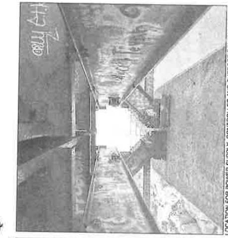
LOCATION FOR POWER SUPPLY, CONTROLLER AND SUPPORT EQUIPMENT ELECTRICAL LIGHTING WILL BE ATTACHED TO THE BEAMS THAT ARE UNDER THE BRIDGE. THE BEAMS ON ONE SIDE OF THE PIER - OTHER SIDE SECURED FOR EQUIPMENT SAFETY.
