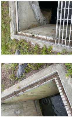
Both grate structures on Foxtrot Taxiway side have 2" inset lip that supports the current aluminum grate.
