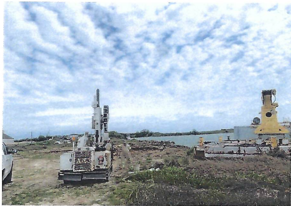
No. 1 View of SB-1 location at the north side of the site.
