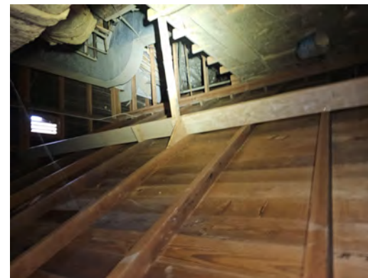
No positive connections of the post supporting the roof beams
