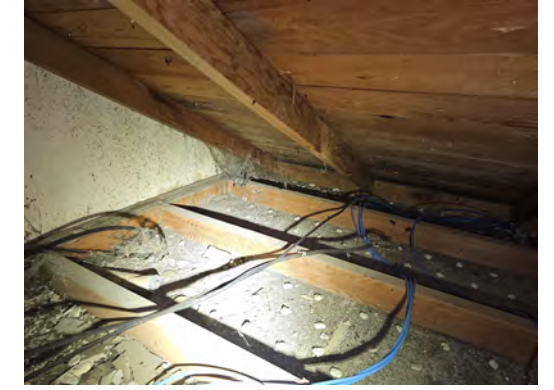
No shear transfer between the roof/ceiling diaphragm and shear walls
