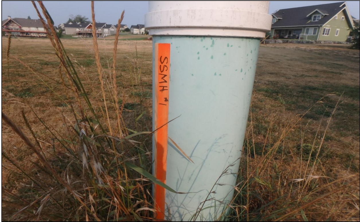
Photo 2. Detail view of the Sewage Line tie-in, view to the west-northwest. Note the Spring Meadows Drive subdivision in the background.
