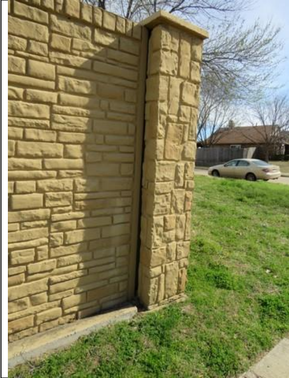
Figure 17 - Panel 1 at exterior of 4129 Stinwick Lane. Panel separated from column.
