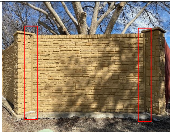
Figure 33 - Panel 1 out-of-plumb and separated from column channel at both sides (annotated by Lerch Bates).
