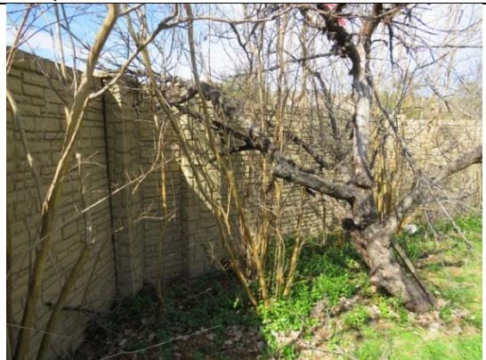
Figure 10 - Tree growth at base of wall adjacent to monument sign panel and at columns.
