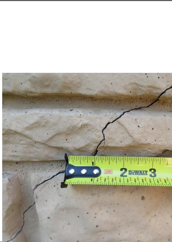
Figure 22 - Enlarged view of crack in Figure 21.
