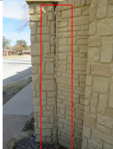
Figure 4 - 2-foot panel section at north end of monument sign, separation from column channel (annotated by Lerch Bates).
