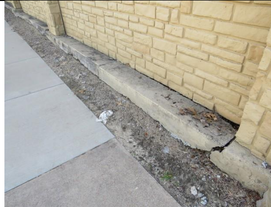
Figure 6 - Cracks and separation at mow strip and column foundation.
