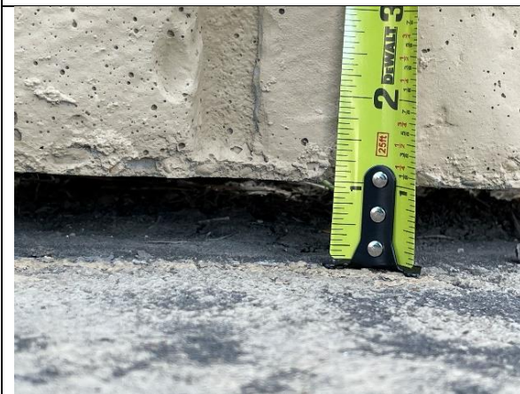
Figure 23 - 1-inch separation at base of panel and mow strip at panel 18.
