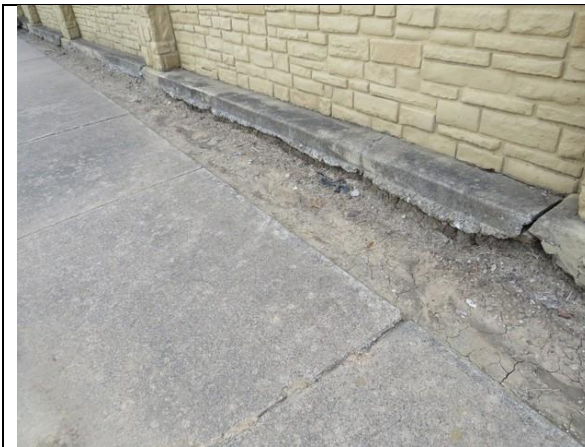
Figure 11 - Typical condition of mow strip along wall.
