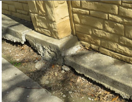
Figure 39 - Typical condition of mow strip along wall and column foundation at wall section 4.
