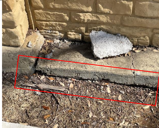
Figure 35 - Exposed rebar at mow strip of panel 3 (annotated by Lerch Bates).
