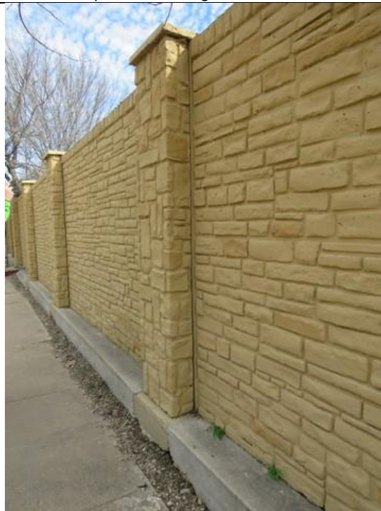
Figure 16 - Previous repair at mow strip along panels 35 through 62 .
