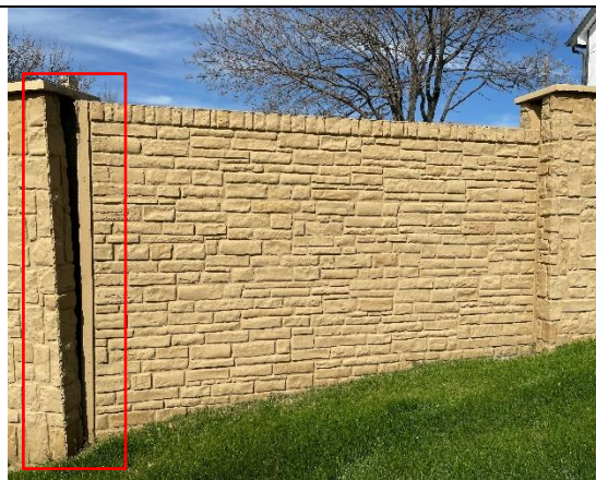
Figure 37 - Panel 3 out-of-plumb and separated from left column channel (annotated by Lerch Bates).
