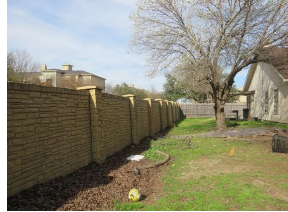
Figure 31 - Debris adjacent to base of wall at the yards of residences 4121 through 4117 Stinwick Lane.
