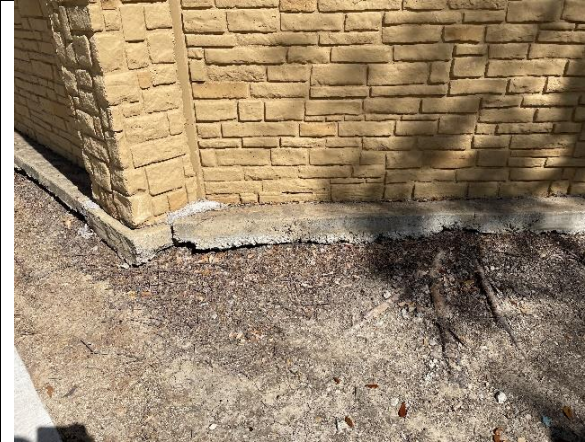
Figure 34 - Protruding tree roots visible at panel 1.
