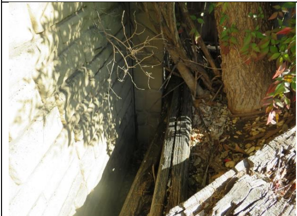
Figure 27 - Tree at corner of panel 41 adjacent to deteriorated wood wall.
