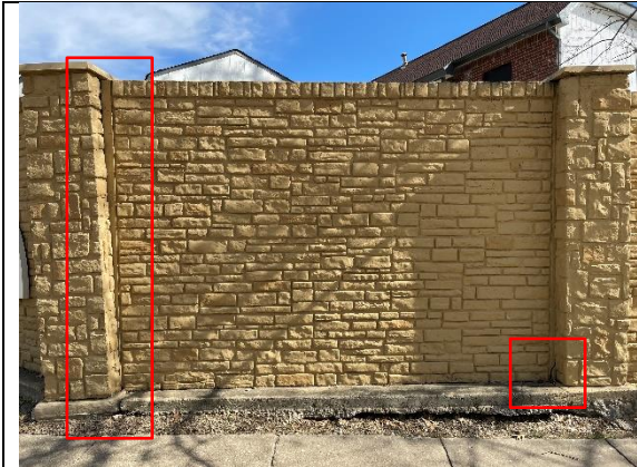
Figure 38 - Panel 8 out-of-plumb and separated from right column channel. Crack is located at bottom right of panel (annotated by Lerch Bates).
