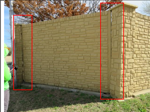
Figure 19 - Exterior view of panel 6 at wall section 2. Panel separated from columns (annotated by Lerch Bates).
