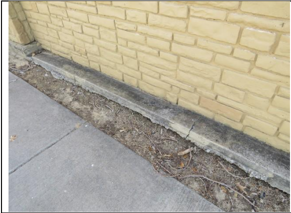
Figure 7 - Cracks and soil erosion at mow strip.
