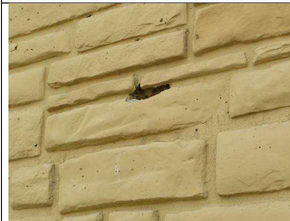
Figure 29 - Void in wall at panel 10.
