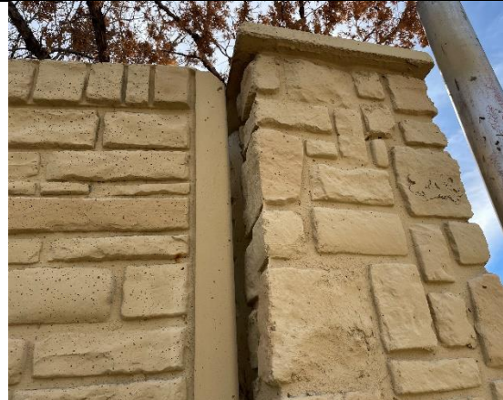
Figure 20 - Exterior view of panel 7 at wall section 2. Panel separated from column.
