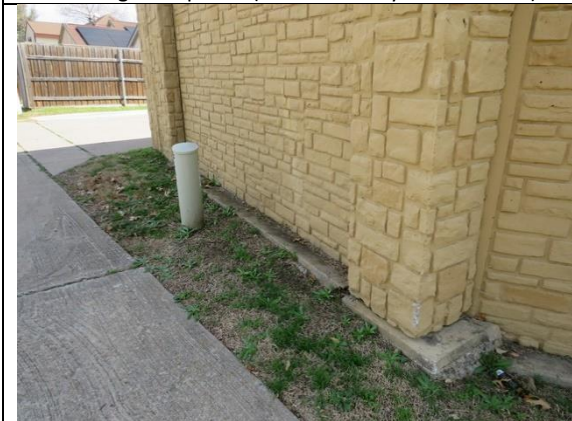
Figure 40 - Typical condition of mow strip along wall and column foundation at wall section 4.
