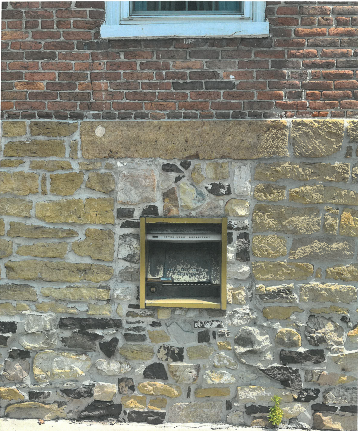
LOCATION OF NEW ENTRY DOOR IN LOCATION ALREADY ALTERED BY PREVIOUS BANKING INSTITUTION.
