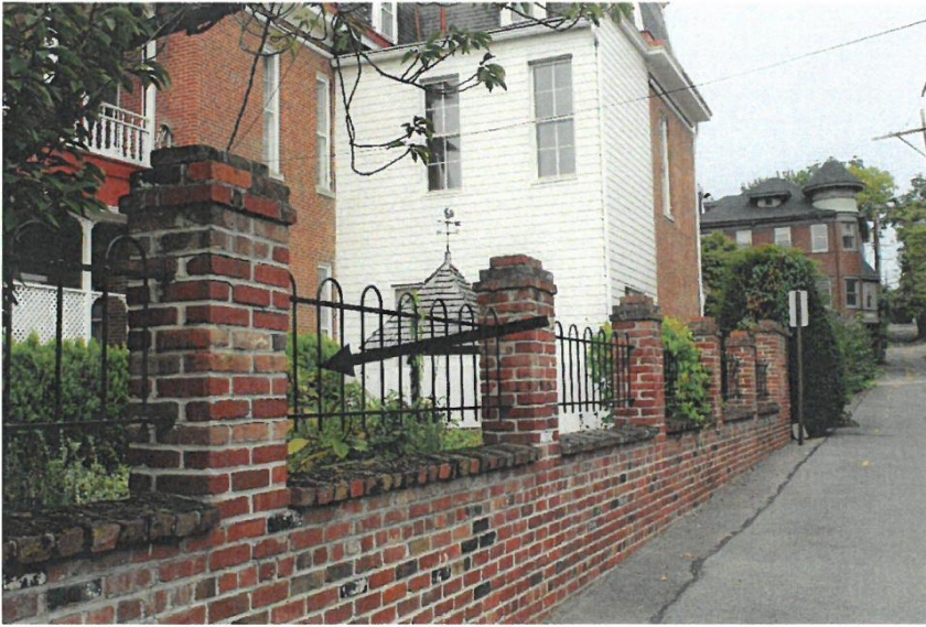
Pier 5 shows some broken mortar, facing northwest.
