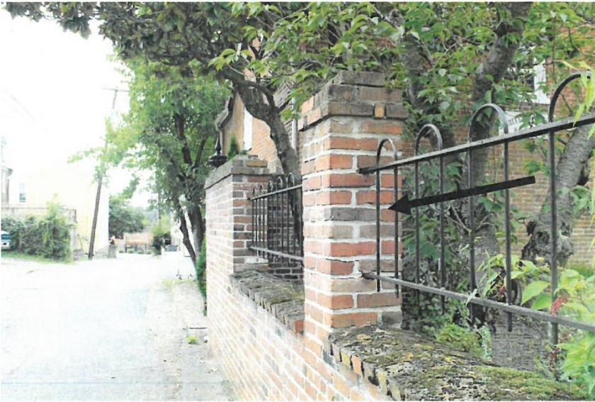
Pier 5 is not as badly cracked as others but still is splitting where the metal railing is attached, facing south.
