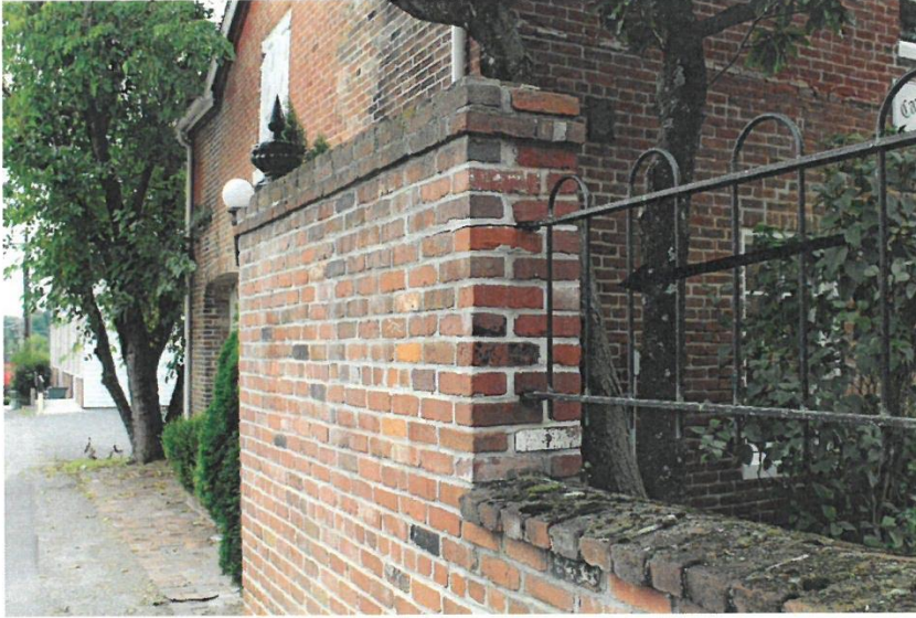
South end cap wall has split mortar but is stable and not in danger of toppling, facing southwest.
