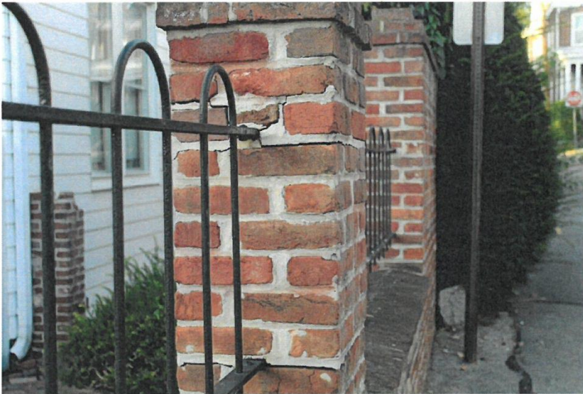
Pier 1 with the mortar cracked where the metal enters the brick piers, facing north.
