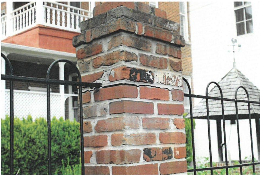
Pier 4 is cracked all the way around and barely holding together, facing northwest.
