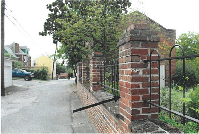
Pier 3 with cracked mortar where the metal is attached, facing south.
