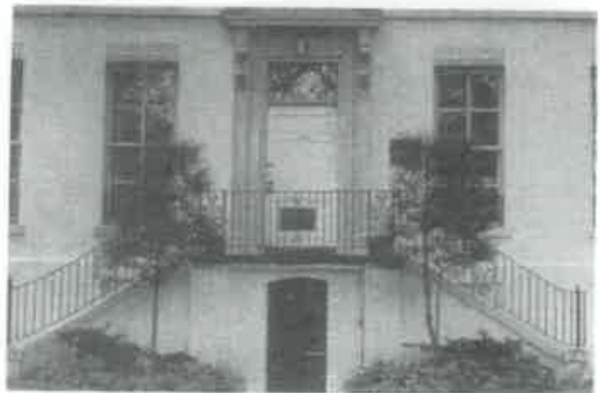
Figure 1. It is important to identify the materials, features, and spaces that should be preserved when planning accessibility modifications. These may include stairs, railings, doors, and door surrounds. Photo: National Park Service files.
