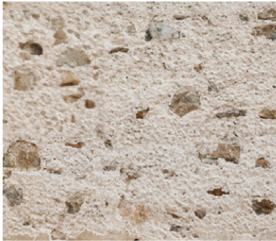
Rubble limestone with heavy mortar smear
