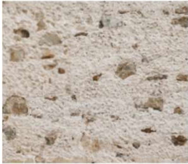
Rubble limestone with heavy mortar smear
