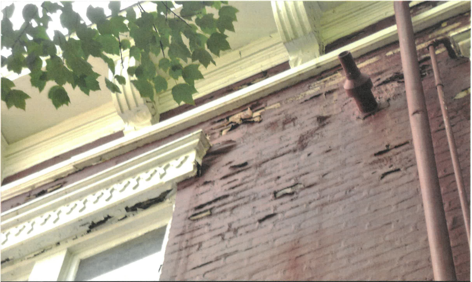
Allegany County Chamber of Commerce (Bell Tower ) Building - Cumberland, Maryland - August 22, 2023 - Photograph by Albert L. Feldstein
