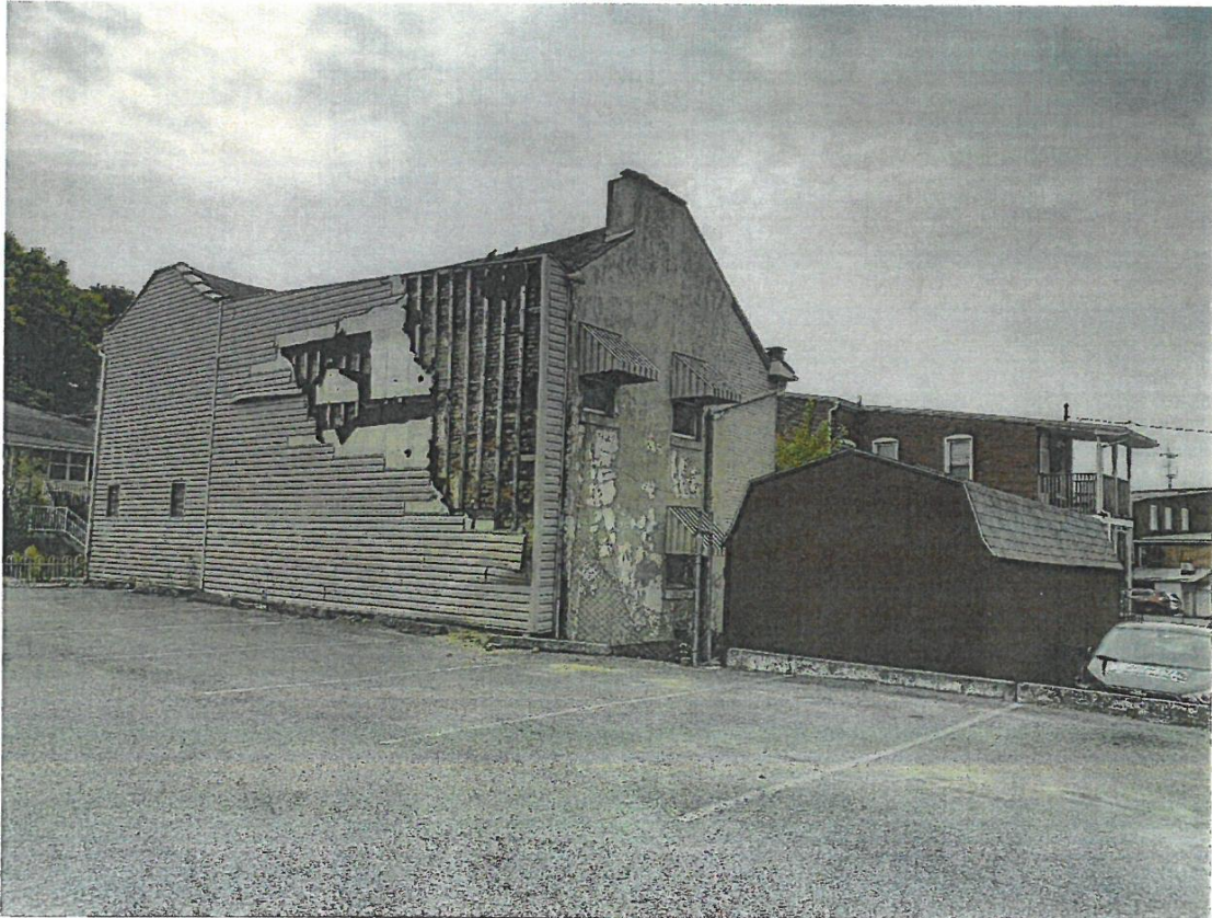
Photo 3 – View of East and North side of dwelling. The exterior brick and the exterior cementitious coating of the brick on the North side of the dwelling is in extremely poor condition.
