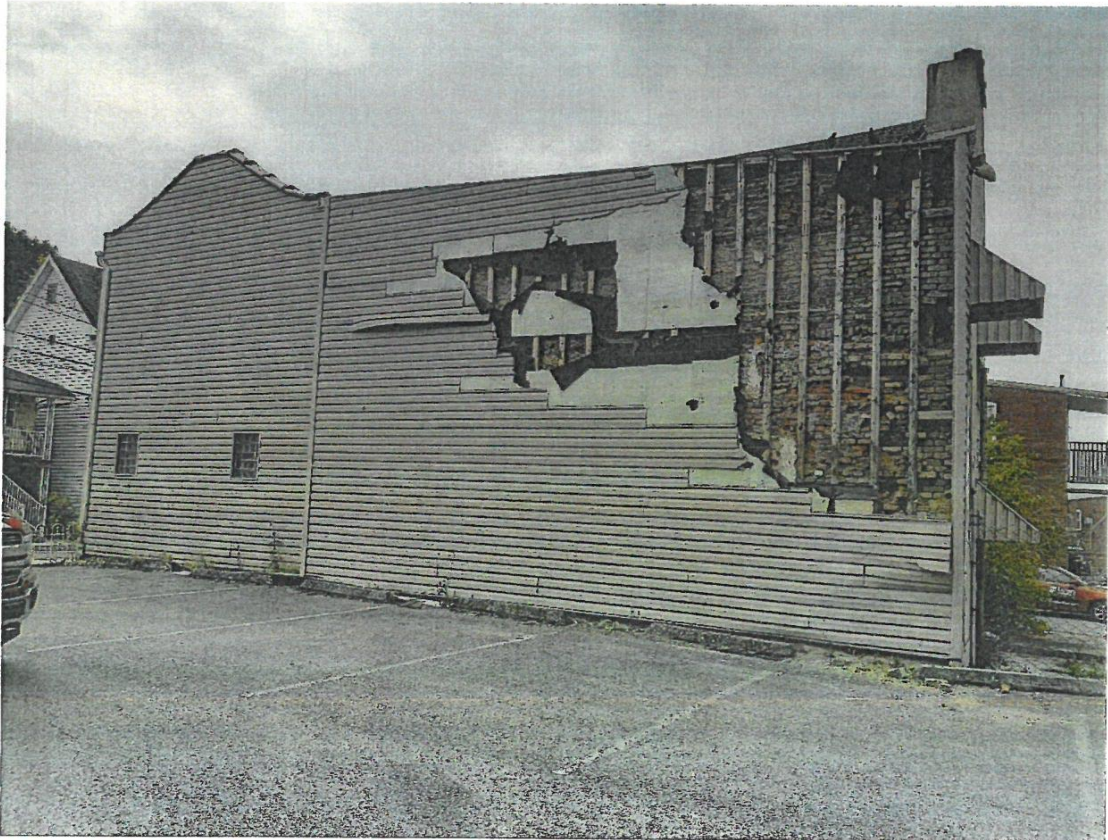
Photo 2 - View of East side of dwelling. Note the brick deterioration on the Northeast corner. The 2x4 furring strips that have siding attached are no longer attached to the deteriorated brick and are in danger of detachment under high wind conditions.
