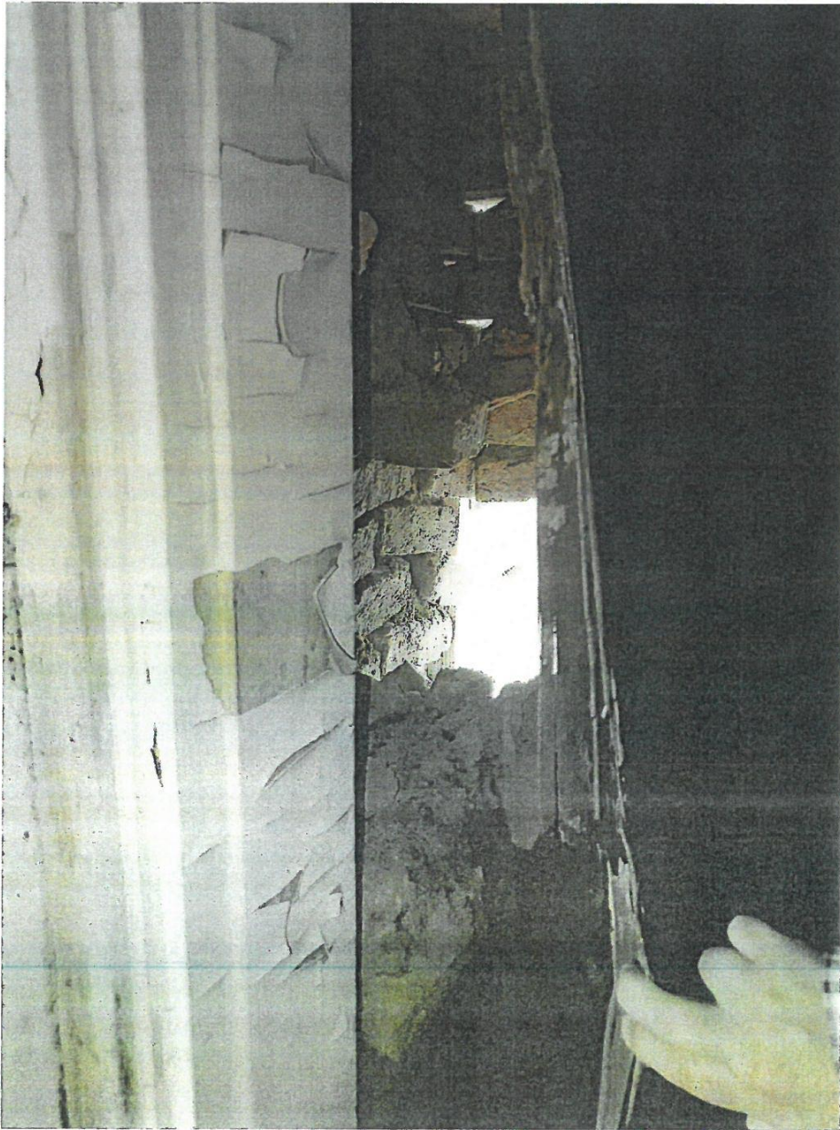
Photo 7 – View of daylight coming through second floor bedroom wall at the Northeast corner of the dwelling.
