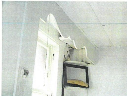
Discoloration on wall in Kitchen
