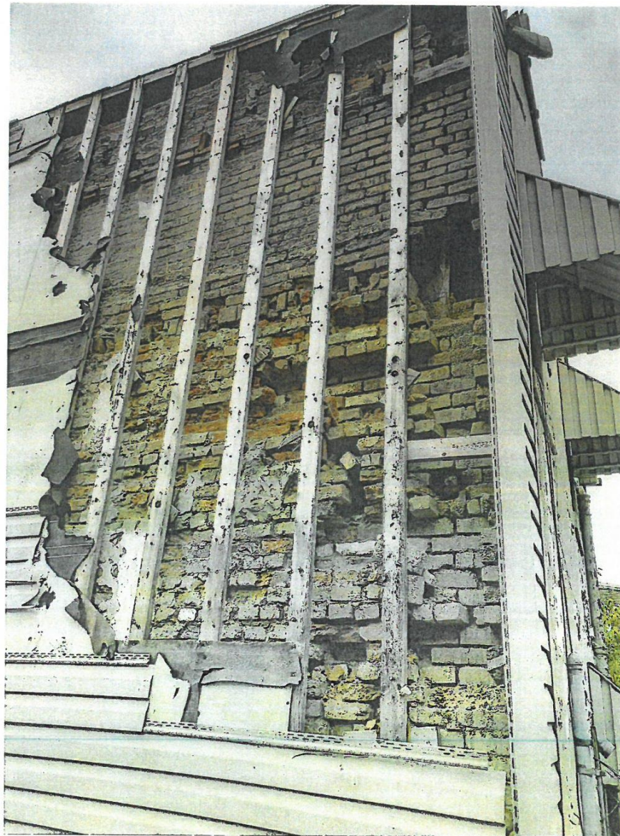
Photo 6 – Closer view of the Northeast side of the dwelling and the extent of brick and mortar deterioration.
