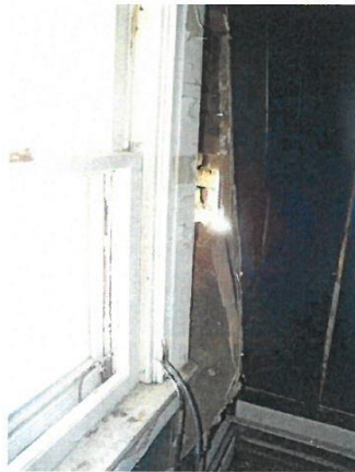
Wall open to outside
