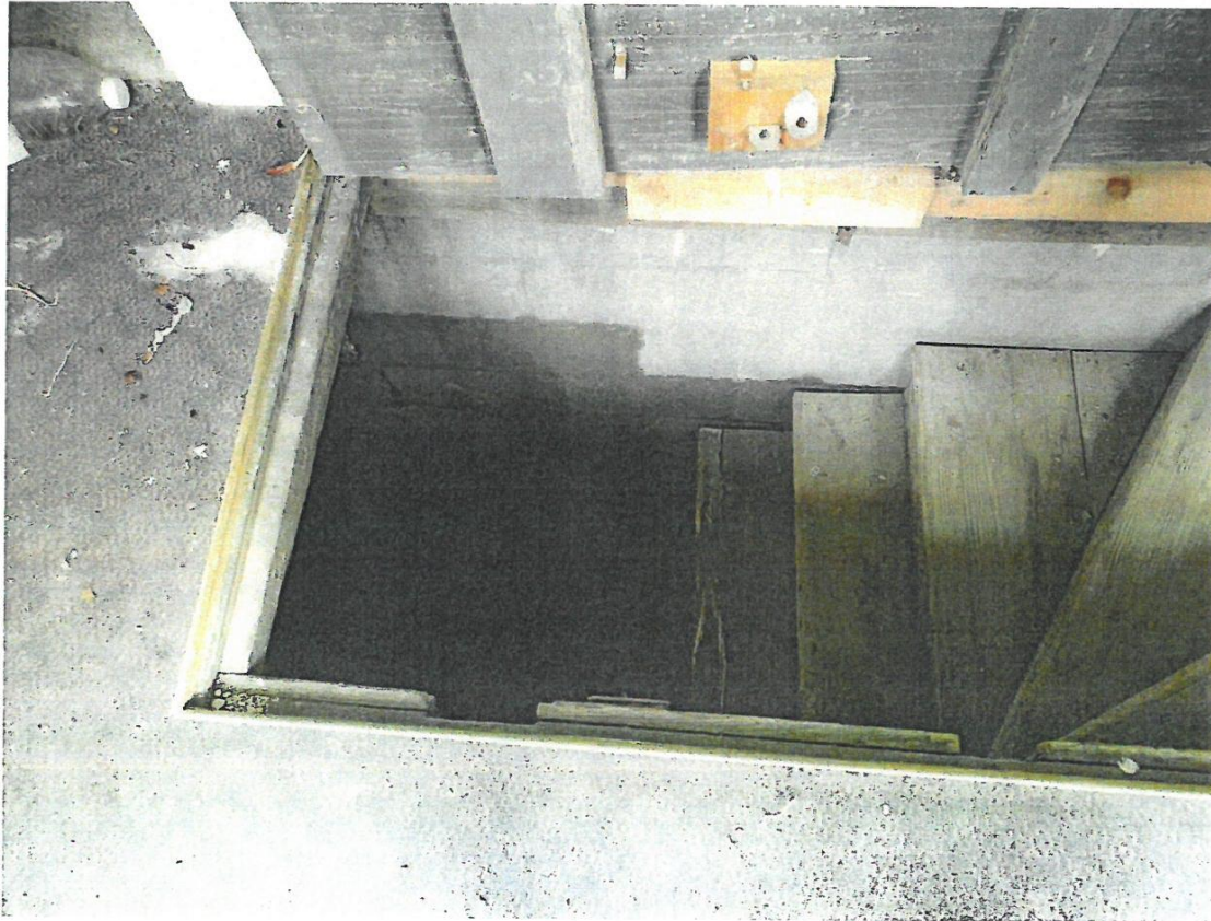
Photo 8 – View of stairs leading to the basement. Note the water stains on the concrete block where the lower standing water has saturated the block by capillary absorption.
