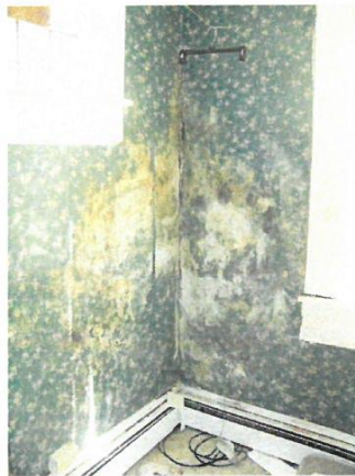
Discoloration on wall in Living Room
