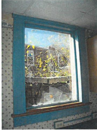
Broken Window in Kitchen
