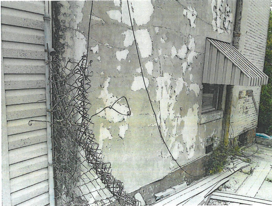
Photo 5 – Closer view of the North side of the dwelling and the cementitious brick coating. Note cracking and delamination of the coating and surface.
