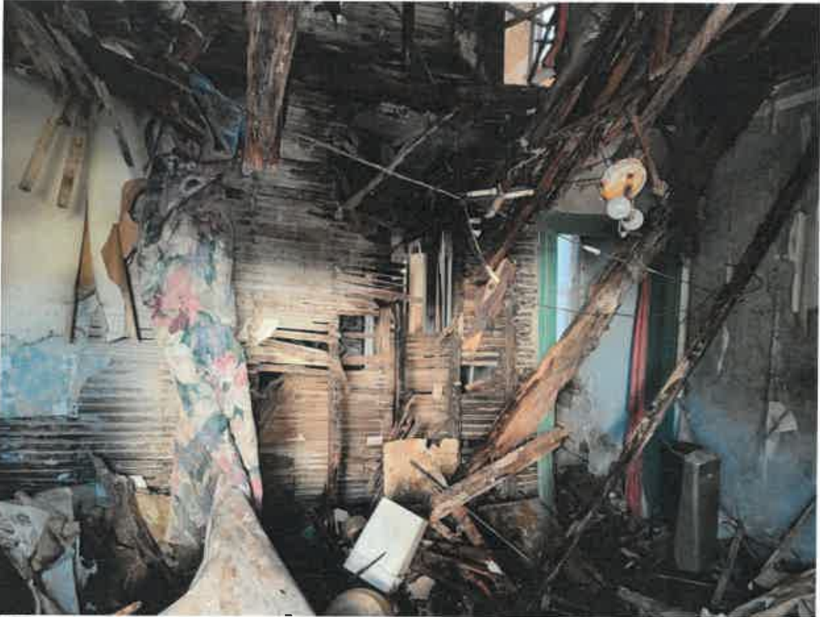
Photo 3. Interior photograph showing current state of disrepair.
