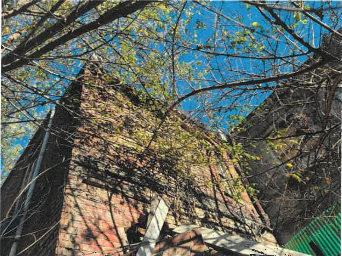
Photo 6. Rear wall. The entire wall is bowed out and the top of the wall is already caved in. Note the opening at the lower part of the photo- this is the door to the rear with the brick falling out.
