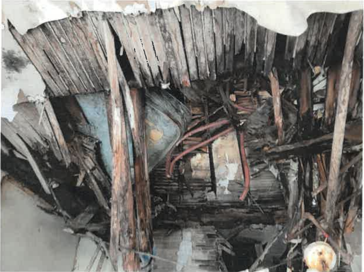
Photo 4. This part of the roof that has collapsed through the upper floor.
