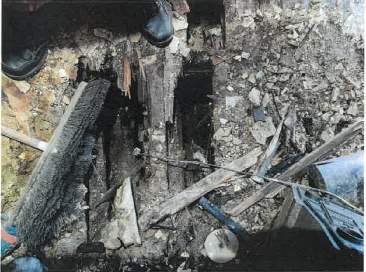
Photo 5. This is looking through a hole in the first floor to the basement.
