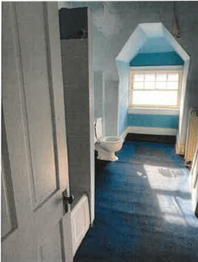
Apartment 5. Floor to be refinished, new water-efficient toilet installed, new tile for tub-surround.
