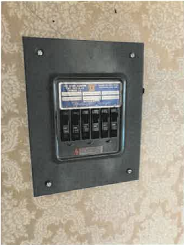
2 nd Floor service box encompassing non-grounded wiring to be replaced at re-wire.
