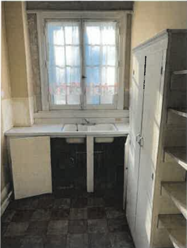
Apartment 3. New counter and sink. New electric stove and fridge. Sand and refinish floor.
