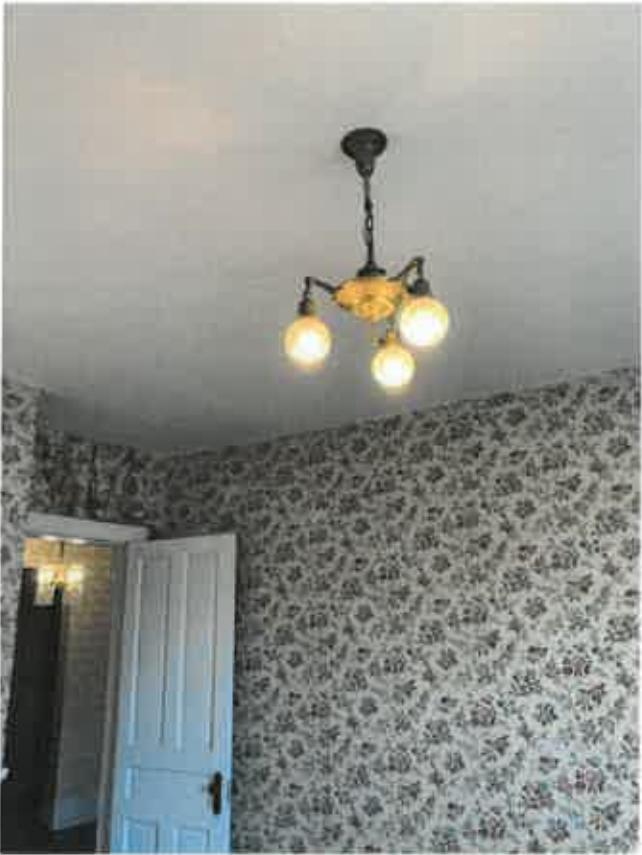
Apartment 3 living room. Plaster and wallpaper patch right side above window.
