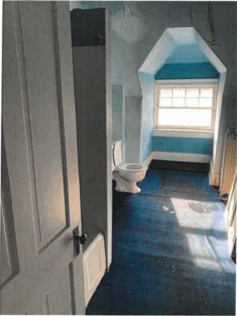
Apartment 3 bathroom carpeting to be removed and original tile floor cleaned and re-grouted.
