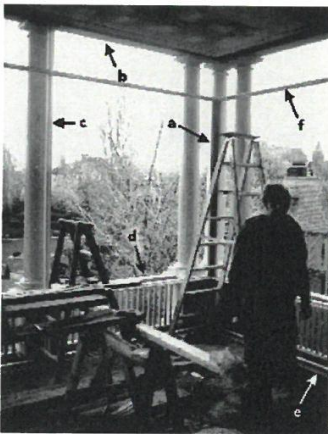
Figure 16. The use of near full glazing to enclose a porch may be appropriate depending upon the historic character of the building, location of the porch, how the interior space is to be treated, and other factors. This enclosure of a rear porch to create a conference room successfully utilizes large expanses of glass and narrow metal framing set behind existing porch elements (a through e). Where an additional horizontal support was needed (f), the frame was placed at a location that is found in many traditional insect screen enclosures. Photo: Charles Fisher.
