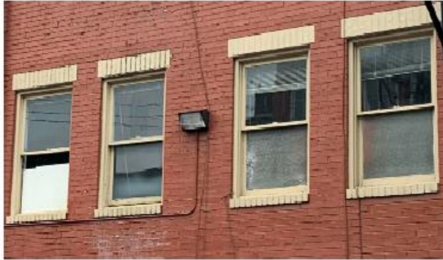
Photo: Additional before pic of mismatched and missing windows #3 Apr 06, 2021
