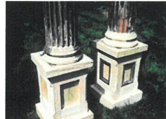
Figure 10. This nineteenth century porch column is made of wood staves, similar to the way a wood barrel is put together. After replacing the torus and making dutchman repairs to the apophyge along the base, the column and pedestal are ready to be reinstalled on the porch. Photos: NPS files.
