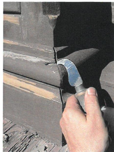
Figure 7. Common problems with porches that can contribute to serious wood decay include cracks in woodwork and joints that have opened up. Both provide an easy path for water seepage. Trapped moisture can foster peeling paint, wood decay and insect infestation. Open joints and cracks should be checked for evidence of more serious decay and marked for caulking or repair. Photo: John Leeke.
