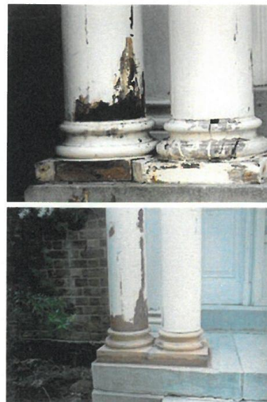
Figure 11. The lower shaft of the porch columns had decayed as water wicked up through the end grain (top). The column shafts were repaired in place by cutting out the deteriorated wood and making repairs using epoxy consolidants and fillers, (bottom). The column bases were replaced. Photos: Paul Marlowe, Marlowe Restorations.
