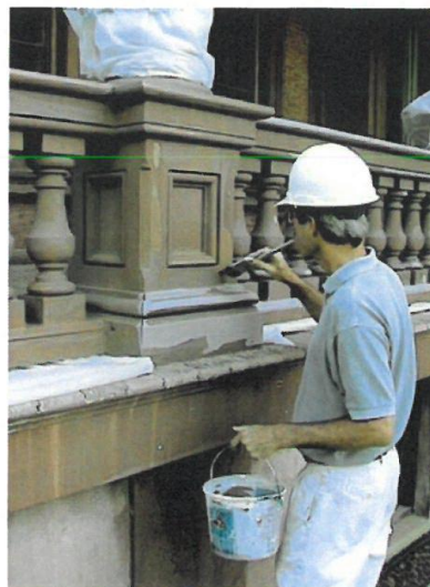
Figure 8. Decay can start when wood is left exposed to the weather or where joints open up. An inexpensive way to extend the life of the existing porch paint without jeopardizing the historic material is spot paint and caulk where needed every year or two. This cost-effective procedure is particularly effective in maintaining wood porches where the exposure to weathering is high. Photo: John Leeke.
