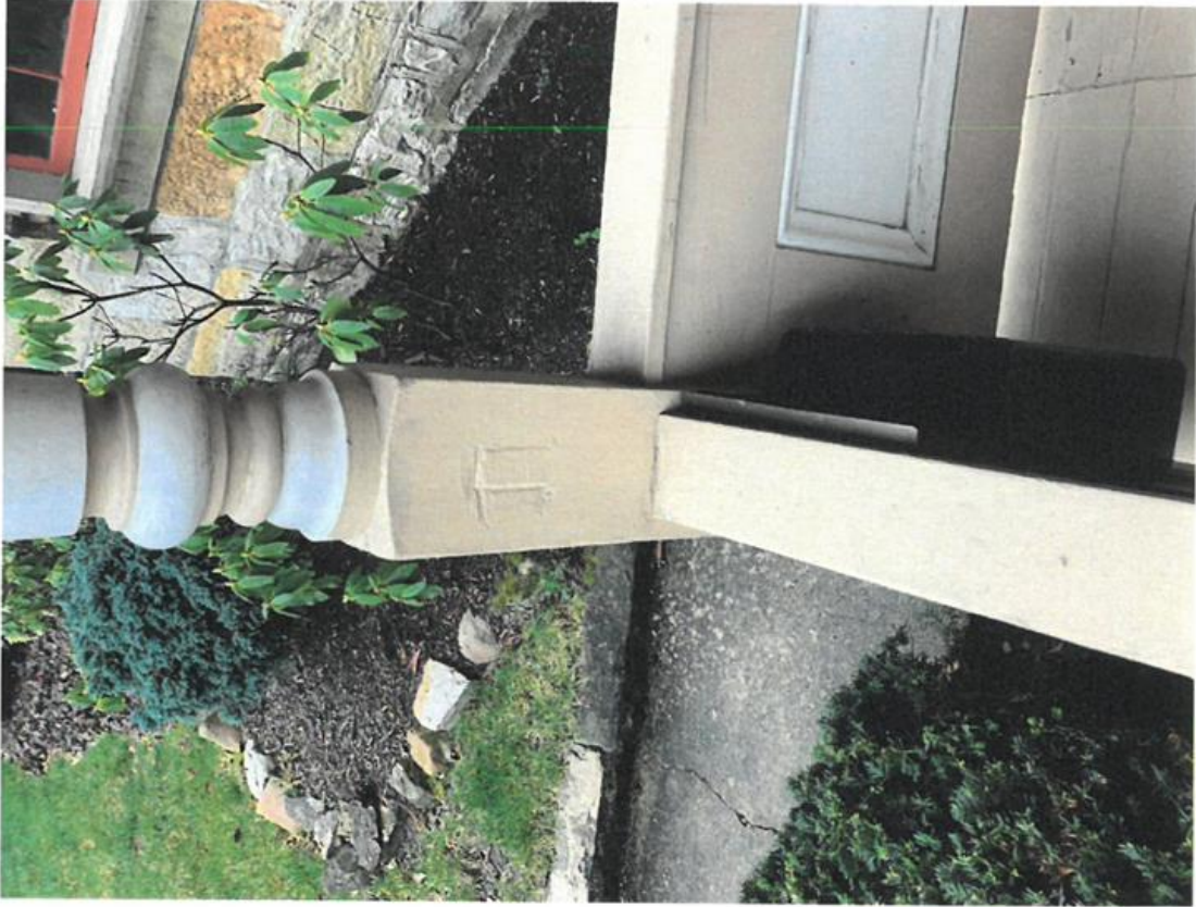
Photo: Front post bottom you can see the cut-off area We want to put the rail back in this location Apr 01, 2021
