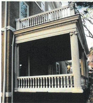
Figure 17. The porch's structural system must be capable of supporting today's loads. In this case moisture led to the deterioration of the wood girder at the corner, creating a major structural deficiency (top). A new solid timber was installed to replace the girder (middle); alternatively a built-up girder could have been used since a fascia board would conceal it. The column base was repaired and portions replaced and the balustrade and column reset and secured (bottom). Photos: Paul Marlowe, Marlowe Restorations.
