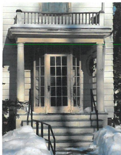
Figure 13. Particularly in New England, there is a cold weather tradition of installing temporary glass and wood panels at entrance doors, thereby creating an enclosed vestibule. These enclosures with their small divided lights were generally removed in the spring. Photo: John Leeke.
