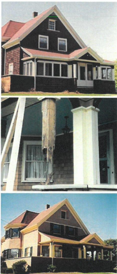
Figure 14. The enclosure of a prominent porch can dramatically change the historic character of a building. The L-shaped porch on this 1896 Shingle-style New England residence was later enclosed with aluminum windows and screens. Recent owners elected to reopen the historic porch. Among the other work, it was necessary to correct structural damage, as with this post, where beneath the wood casing carpenter ants had done serious damage. In reopening the porch, the historic character of the residence has been brought back and the traditional use of the porch is once again enjoyed. Photos: Mark Landry, Landmark Services.
