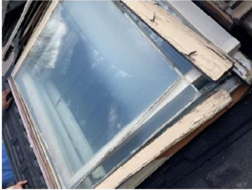
Photo: Additional before pic of rotted/broken windows Apr 06, 2021
