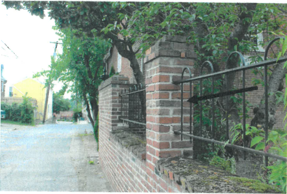
Pier 5 is not as badly cracked as others but still is splitting where the metal railing is attached, facing south.
