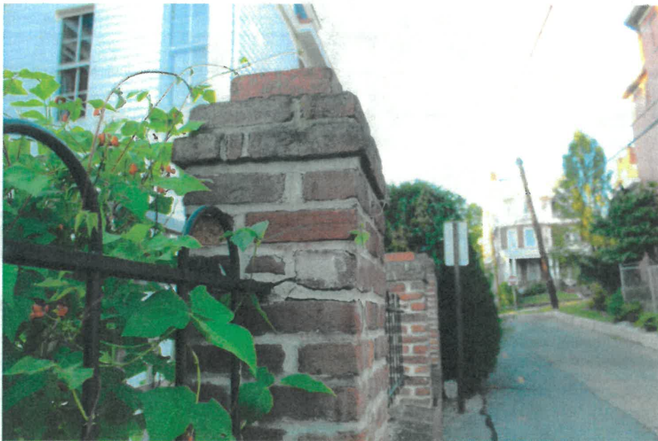
Close up of Pier 2 showing mortar cracks, facing north.
