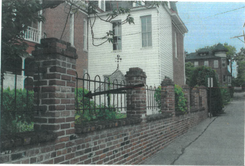
Pier 5 shows same broken mortar, facing northwest.
