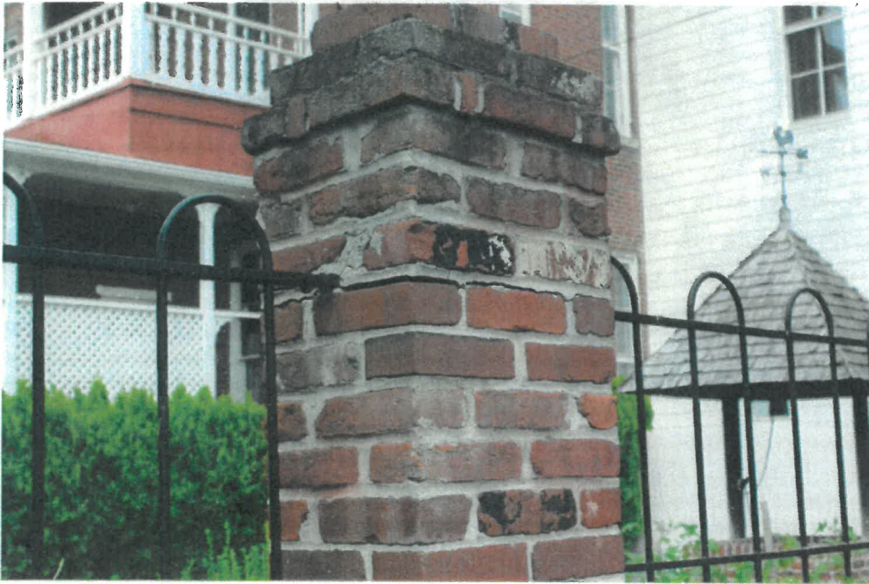
Pier 4 is cracked all the way around and barely holding together, facing northwest.
