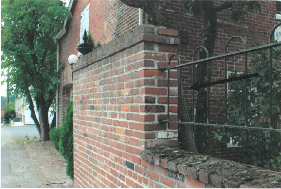
South end cap wall has split mortar but is stable and not in danger of toppling, facing southwest.
