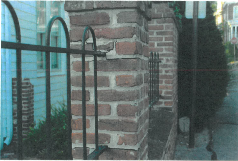
Pier 1 with the mortar cracked where the metal enters the brick piers, facing north.
