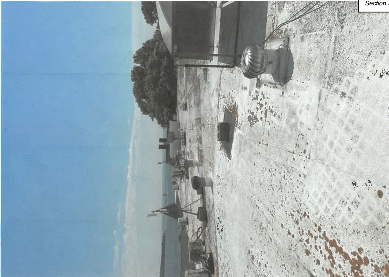
Roof Area Adding AC
