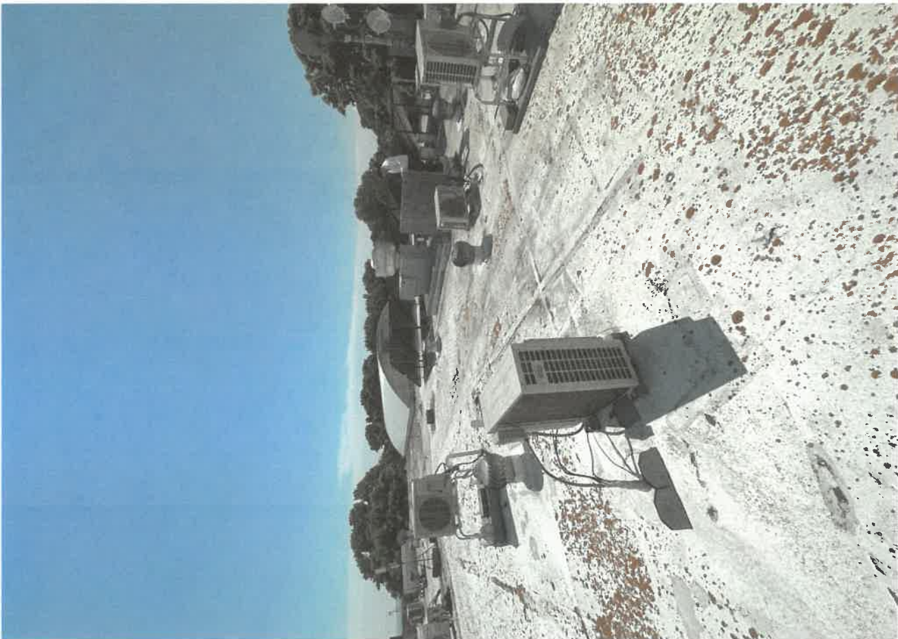
Roof AC units
