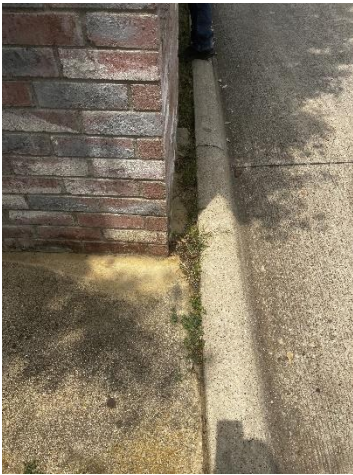
1121-1117 Brevito Dr – Slab Needs Lifting and Top Re-Done
