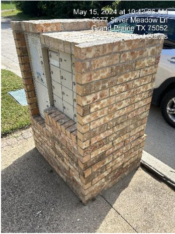
3960-3964 Holly Hill – Slab Lifted
