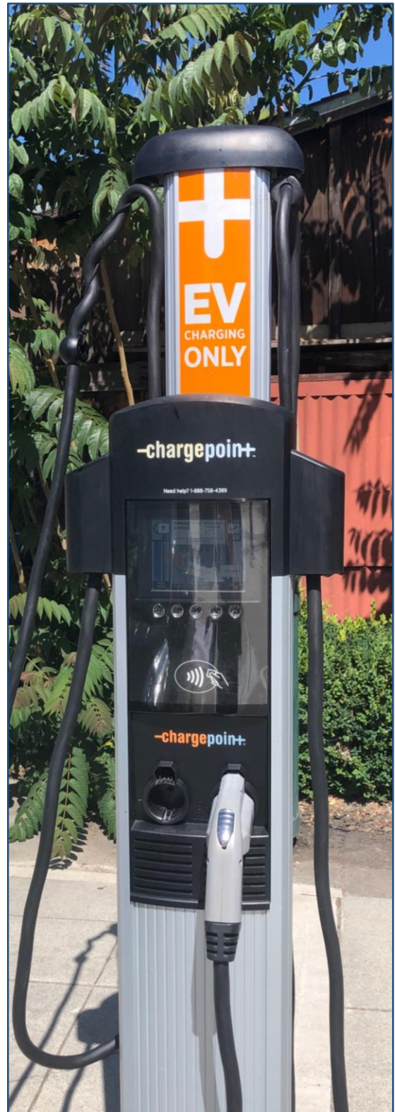
Figure 3: EV Charging Station
