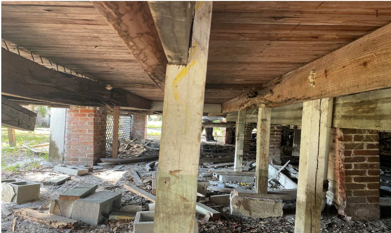
Photo 8: Enclosed Porch Floor Framing – Improper Wood Post/Damaged Floor Joist
