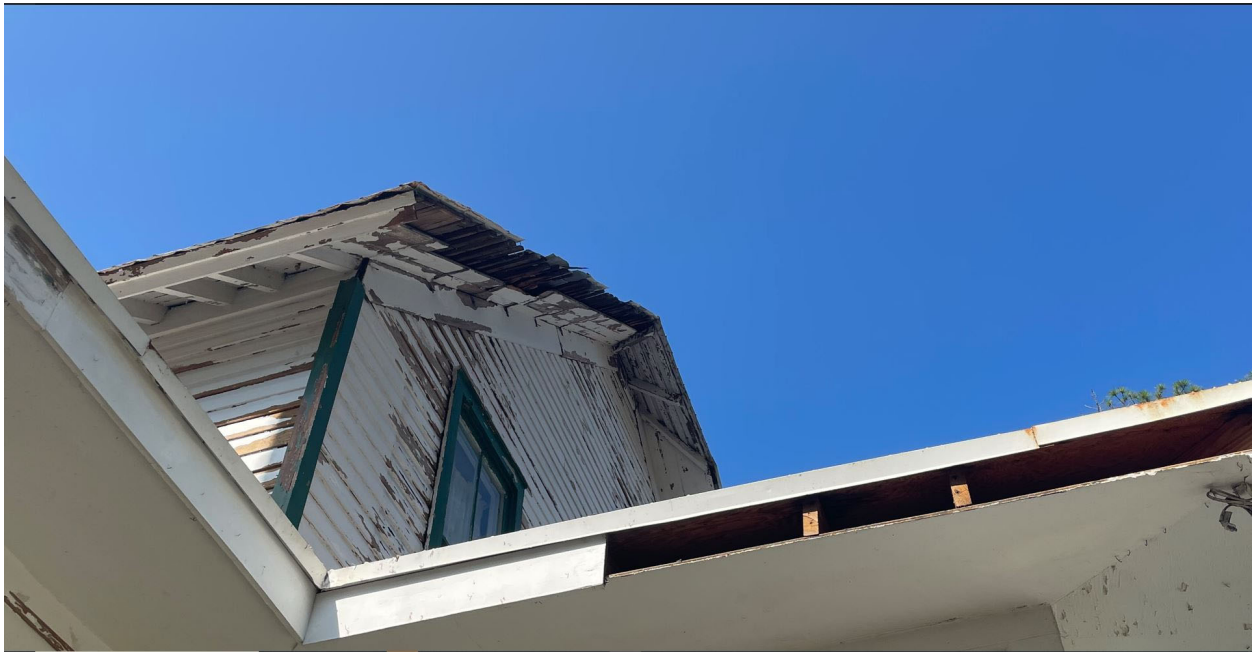
Photo 4: Deteriorated Boards Supporting Metal Roof
