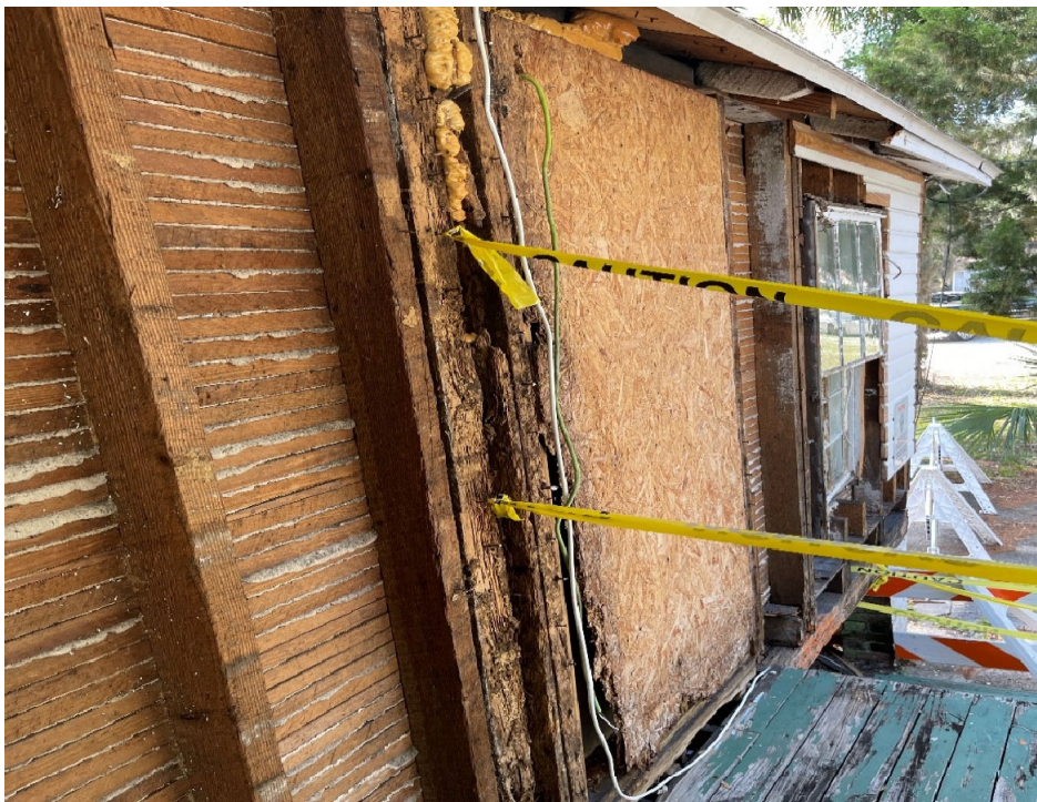
Photo 7: Rear Addition – Damaged Studs
