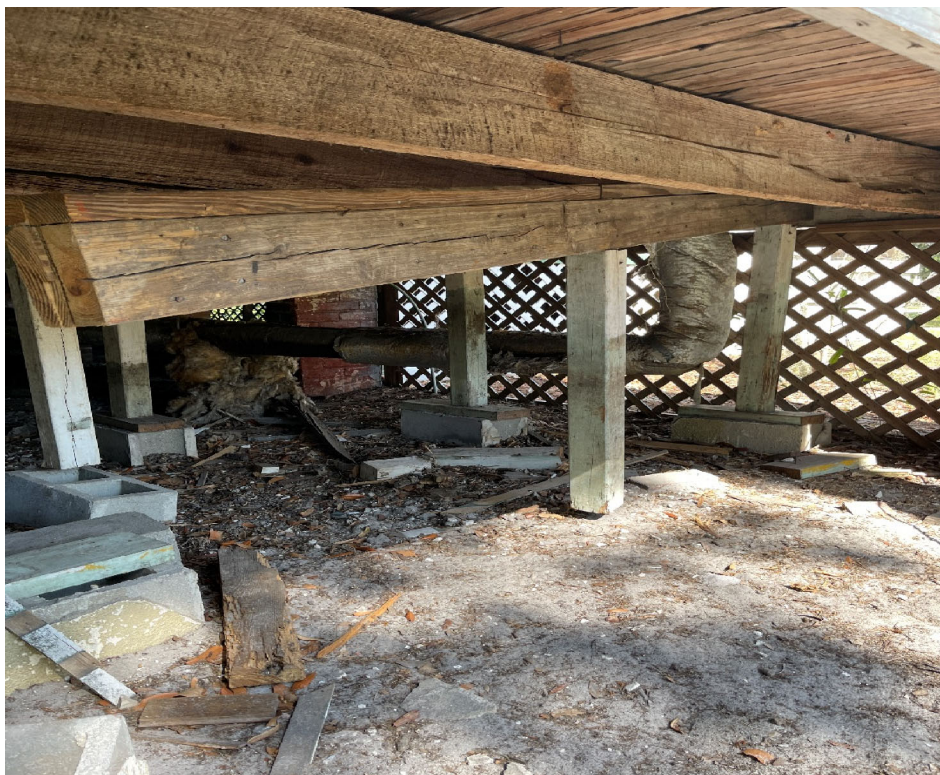
Photo 9: Enclosed Porch Floor Framing – Previous Repair/Unsupported Beam
