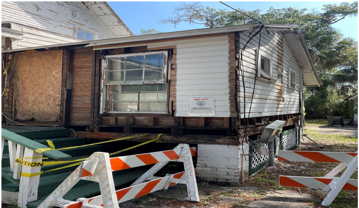
Photo 5: Dilapidated Rear Addition
