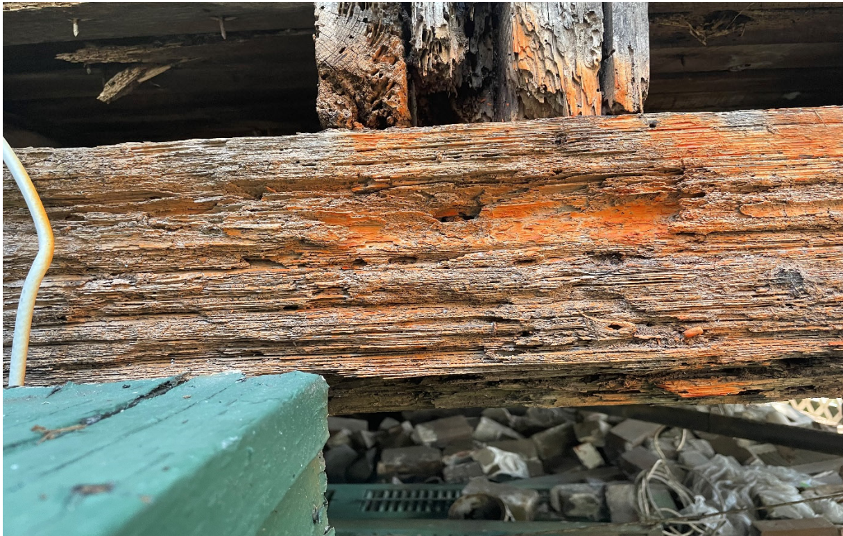
Photo 6: Rear Addition – Deteriorated Perimeter Beam
