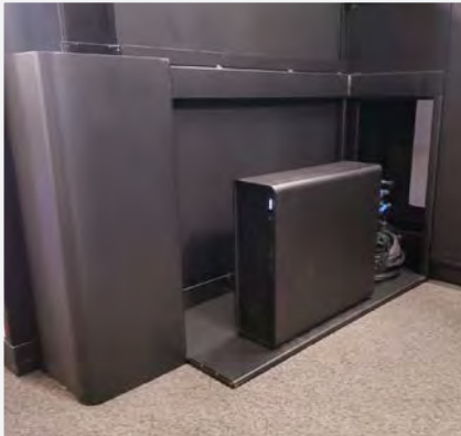
The "L" shaped cover shown removed for maintenance.
