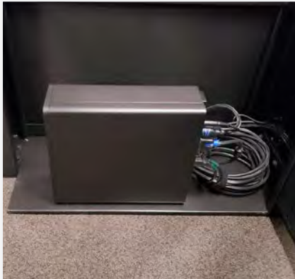
The cabinet houses a mid-sized tower and associated cabling.
