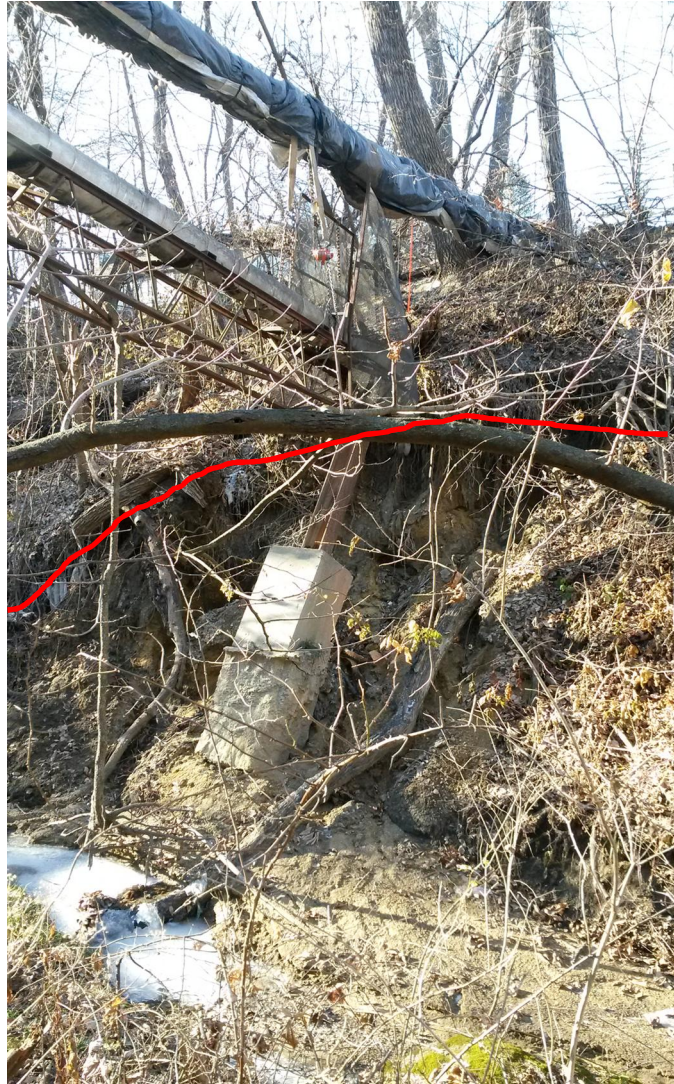
Figure 1 - West ravine slope failure with scarp marked in red
