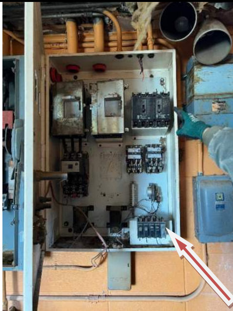
Photograph D-1: Mini-Storage Bldg, pump Rm: Sample 1A black 'Bakelite' electrical switches (about 7 large and 5 small) 30% chrysotile asbestos-containing material (ACM), Category II, non-friable, intact. Orange wall paint contains lead (all paint contains lead).
