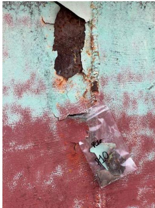
Photograph D-8: Exterior wall of former basin, Sample P10 showing lime paint with red prime contains lead. (Note that all sampled paint contains lead and most also contain cadmium and/or chromium).
