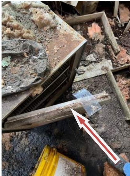
Photograph D-6: Mini-Storage Bldg, Northernmost Rm/lab, white 'rope' packing/gasket around door of old drying oven sitting on floor, contains 55% chrysotile ACM, Category I, non-friable, intact. Pink fiberglass and white ceiling tiles, mostly on floor, do not contain any asbestos.
