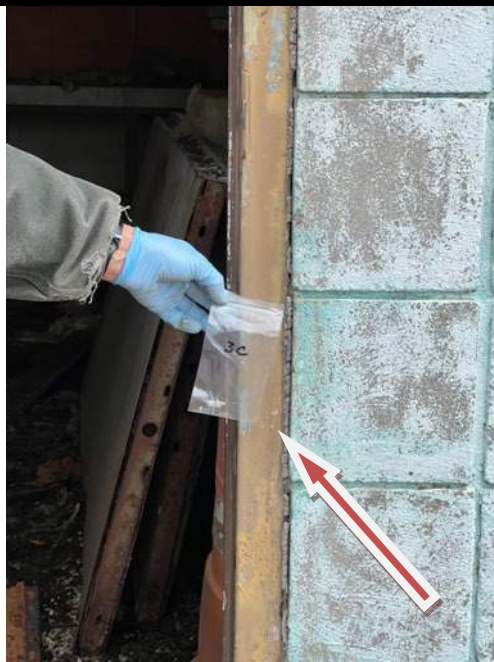
Photograph D-3: Mini-Storage Bldg. Exterior west door to pump room: Sample 3C of Tan/gray door caulking (metal frame to CMU/concrete ext. wall) contains damaged 3-4% chrysotile ACM, Category II, non-friable, damaged. Lime prime paint on frame and CMU walls contains lead.
