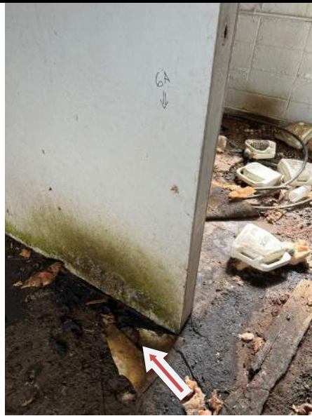
Photograph D-5: Mini-Storage Bldg. Northernmost room; Sample 6A (similar to 6B & 6C) tan floor tile contains 2% ACM, Category I, non-friable, damaged – assume ACM floor tile on all interior flooring. Yellow mastic does not contain any ACM. Floor covered in dirt, mud, carpeting, and debris. While paint on east CMU wall contains lead.
