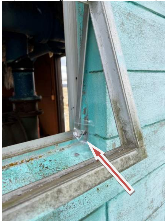
Photograph D-2: Mini-Storage Bldg. Exterior window of pump room, north side: Sample 3B (similar to 3A & 3C) of Tan/gray window caulking (metal frame to CMU/concrete ext. wall) contains damaged 3-4% chrysotile ACM, Category II, non-friable, damaged. Lime paint on CMU walls contains lead.
