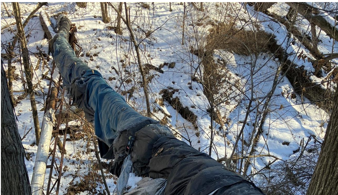
Picture from Friday, February 10 th , 2023 of the Collapsed aerial line (left), and the tarped temporary line attached to a temporary utility pole (center).
