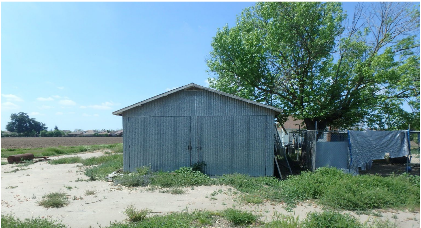
Description of Photo: East façade of corrugated metal storage shed, looking west.
