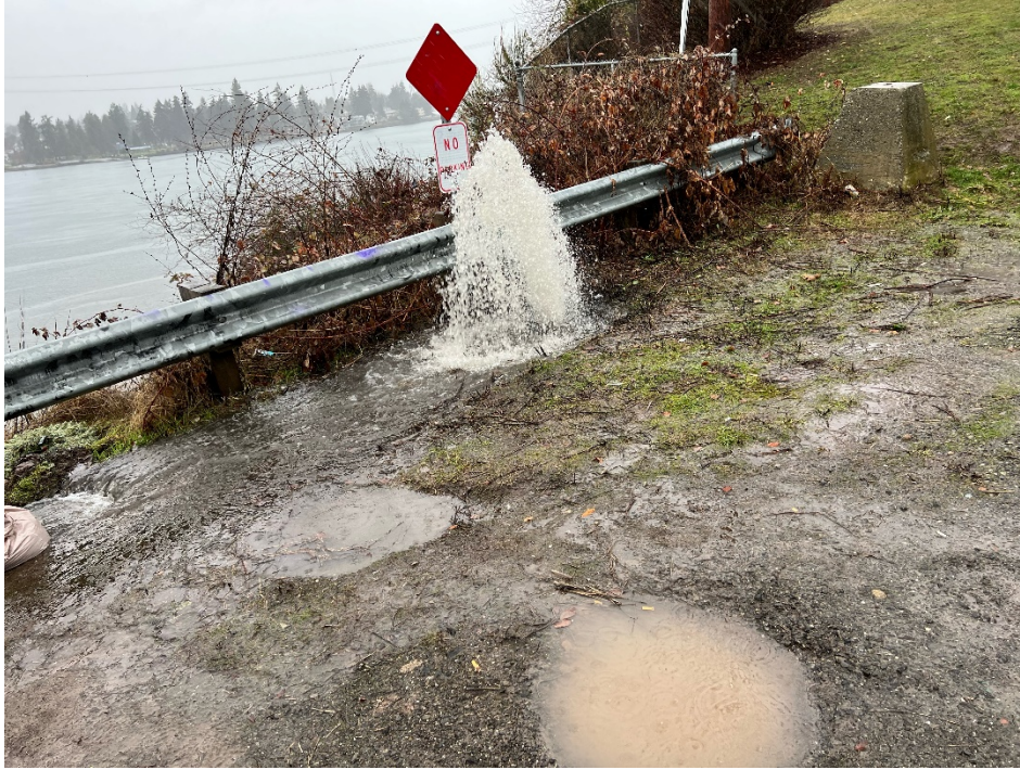
December 24, 2022, stormwater overflow and stream running toward 1717 E 16 th Street.
