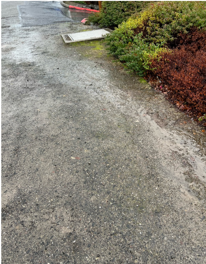
Stormwater running uncontrolled along the south side of the dead end of East 16 th Street
