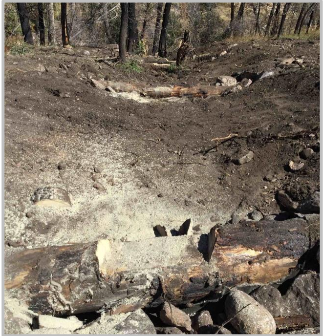
Figure 7: LWM Stabilization installation constructed in the Fall of 2021 in the CLP watershed.
