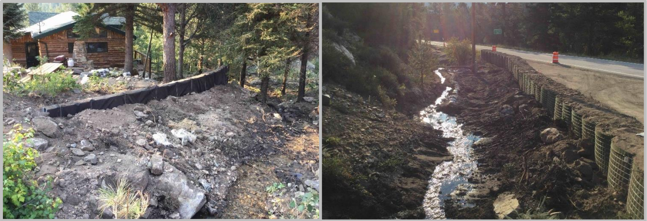
Figure 11: Structure & Road Overtopping Protection at Dry Creek. The area will be stabilized with native vegetation Fall 2021.
