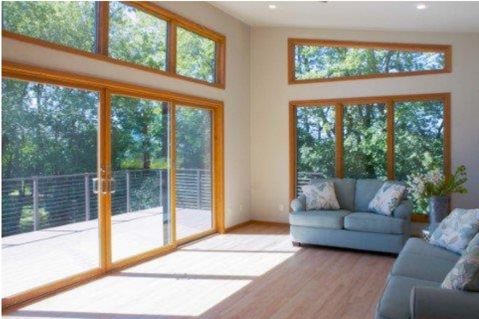
A screened porch was demo'd and a 4-season sunroom with a 16' Andersen patio door installed in this contemporary porch conversion project.
