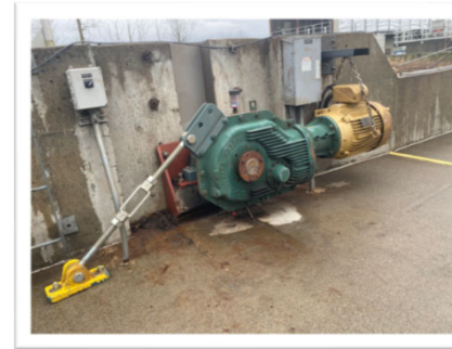
Ditch Rotor Gearbox
