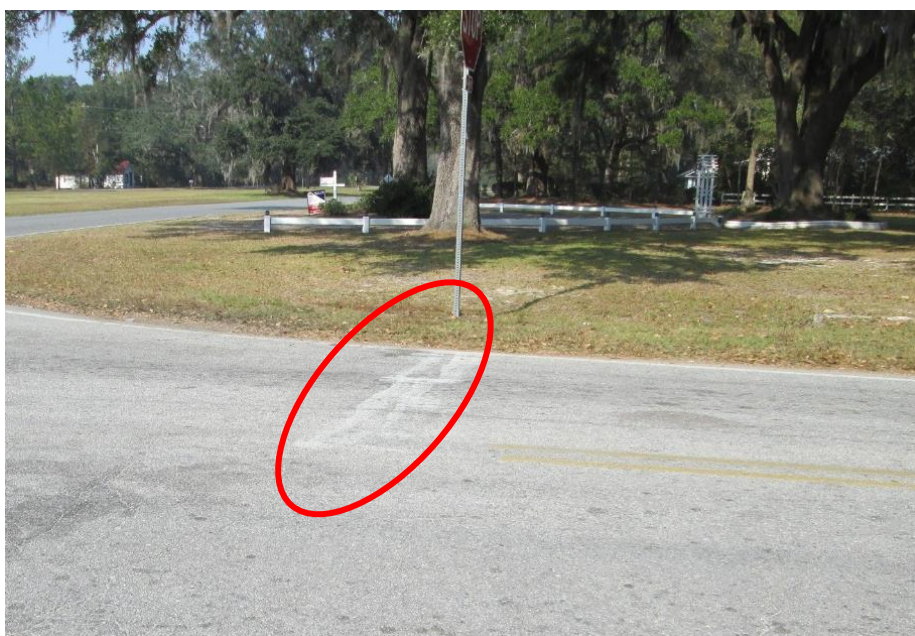
FIGURE 4-6. WORN, FADED STOP BAR AT SANDHILL ROAD AT SANDHILL ROAD/CENTRAL AVENUE INTERSECTION
